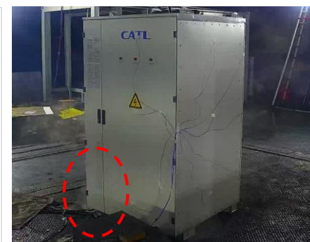
Smoke leakage from rack
