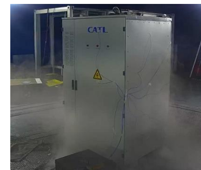
More fumes leakage from rack
